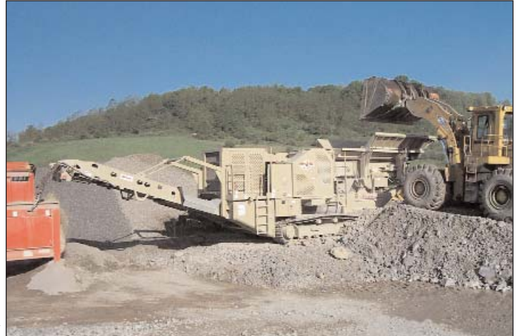
Laurel Aggregates’ President James Laurita chose a track mounted jaw plant for portability onsite, as well as the flexibility to easily move to another site using a low-boy trailer.
